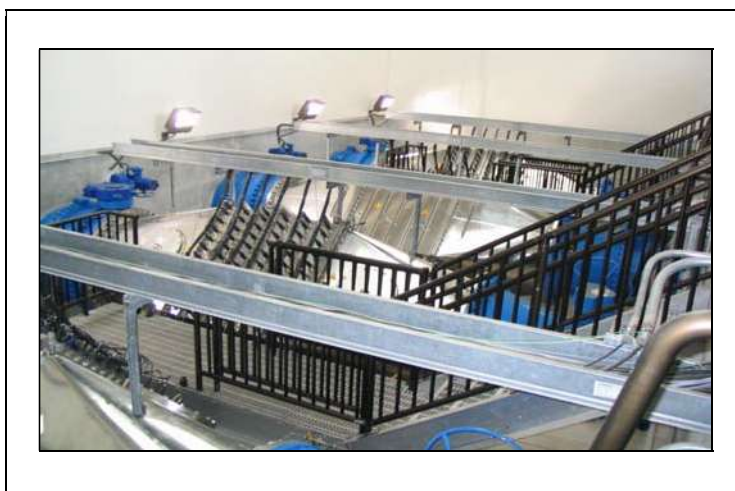
Figure F.13. UV Reactors at the Weber WTP No. 3 (3 duty + 1 standby reactor in parallel)
