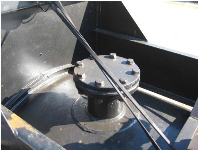
Figure 13 - Torqued bolts not protected
