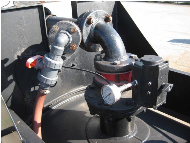
Figure 9- Miscellaneous in-line plumbing not protected
