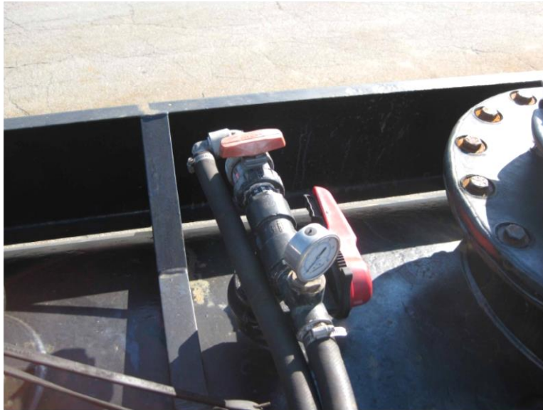
Figure 12- Miscellaneous in-line plumbing not protected
